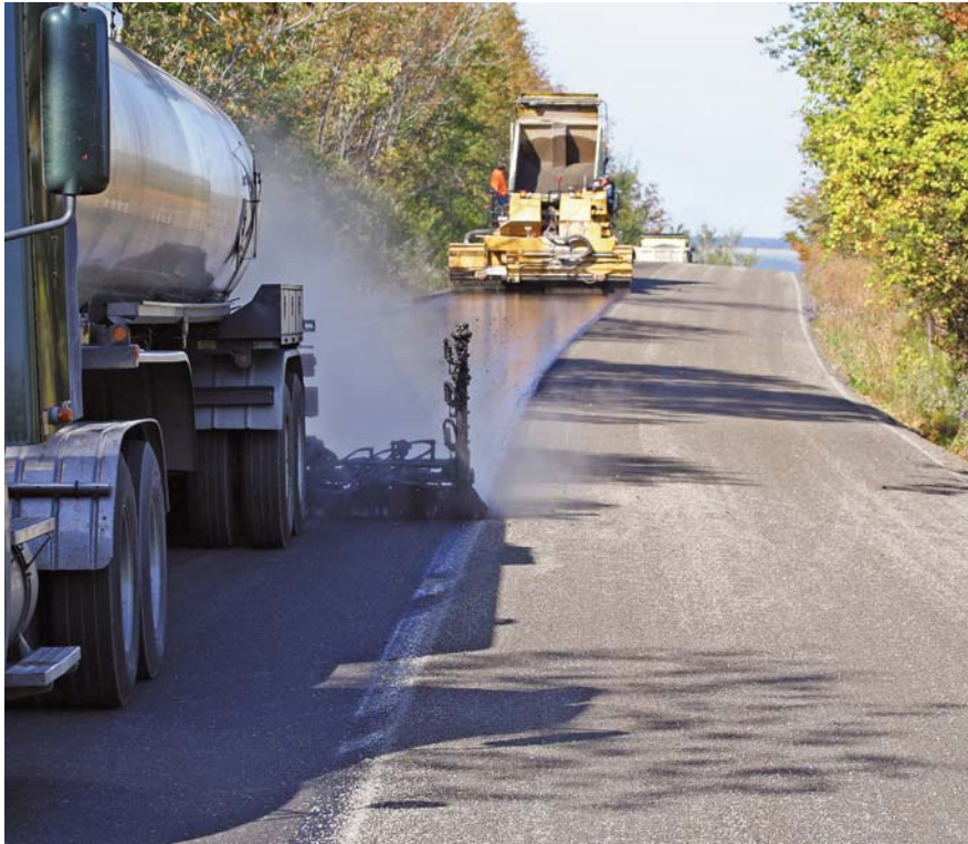
A chip seal wearing course utilizing high-float rapid-set, polymer-modified surface treating emulsion (HFRS-2P) and NYSDOT-approved 1A-sized aggregate was placed.
