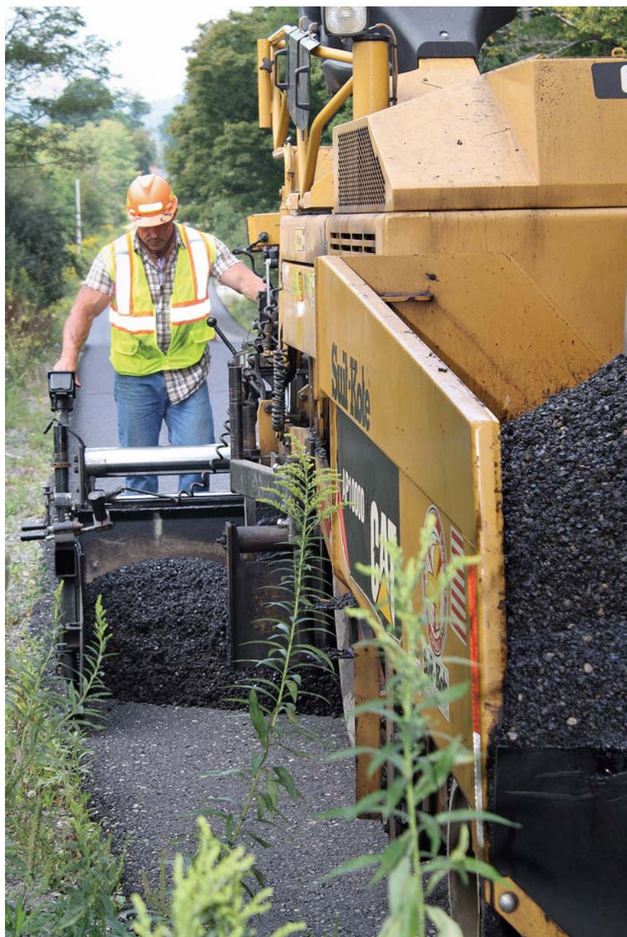
A dense-graded cold mix utilizing a high-float, medium-set, hard-based asphalt emulsion is placed on Truxton-Tully Road in Cortland County, N.Y.
